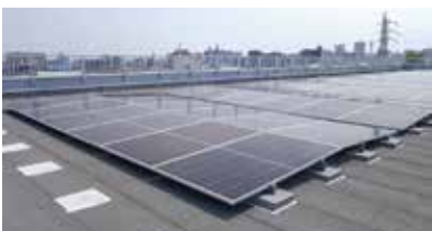
We are actively working to utilize renewable energy, including the installation of solar panels on the headquarters roof.
