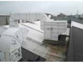
Painting booth exhaust duct
